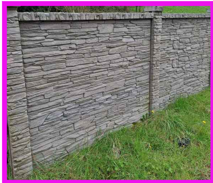
FENCE 1C DESCRIPTION: 8' TALL MODULAR PRECAST STONE WALL COLOR MATCHED TO EXISTING STONE
