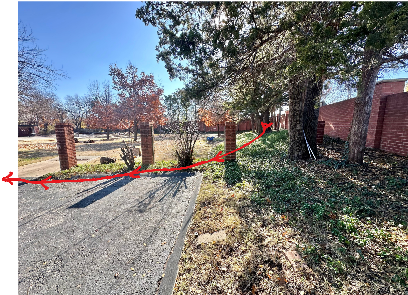
Inside the “walls” exhibiting the “bathtub-like” drainage issues that plague the property without mitigation
