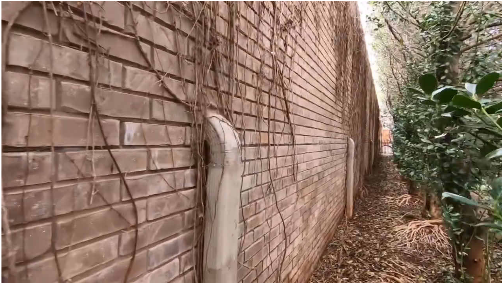
ABOVE: CLOSE-UP OF RETAINING WALL DRAINAGE SYSTEM PRIOR TO COLLAPSE
