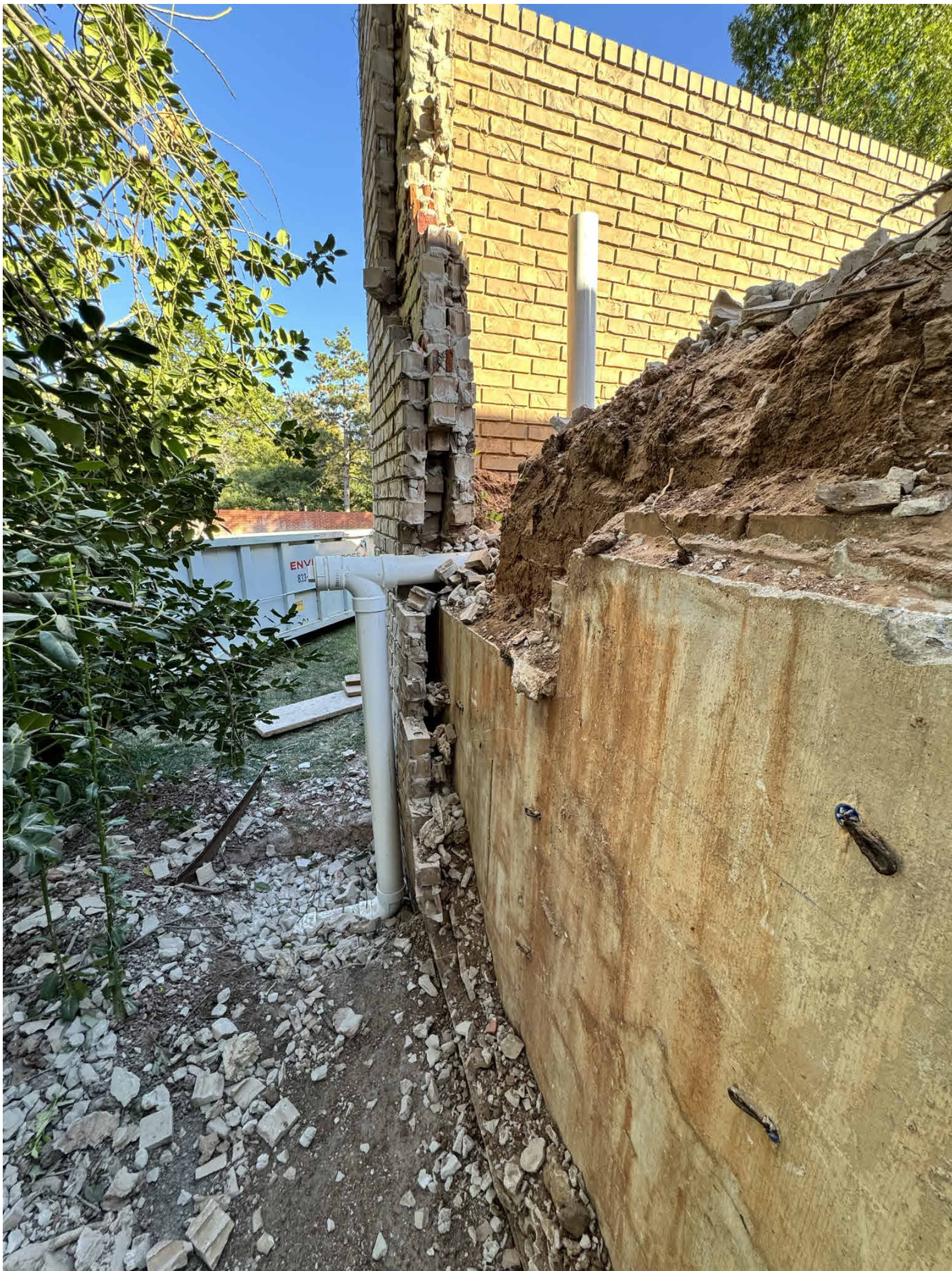
BELOW: RETAINING WALL FAILURE AT GRADE CHANGE
