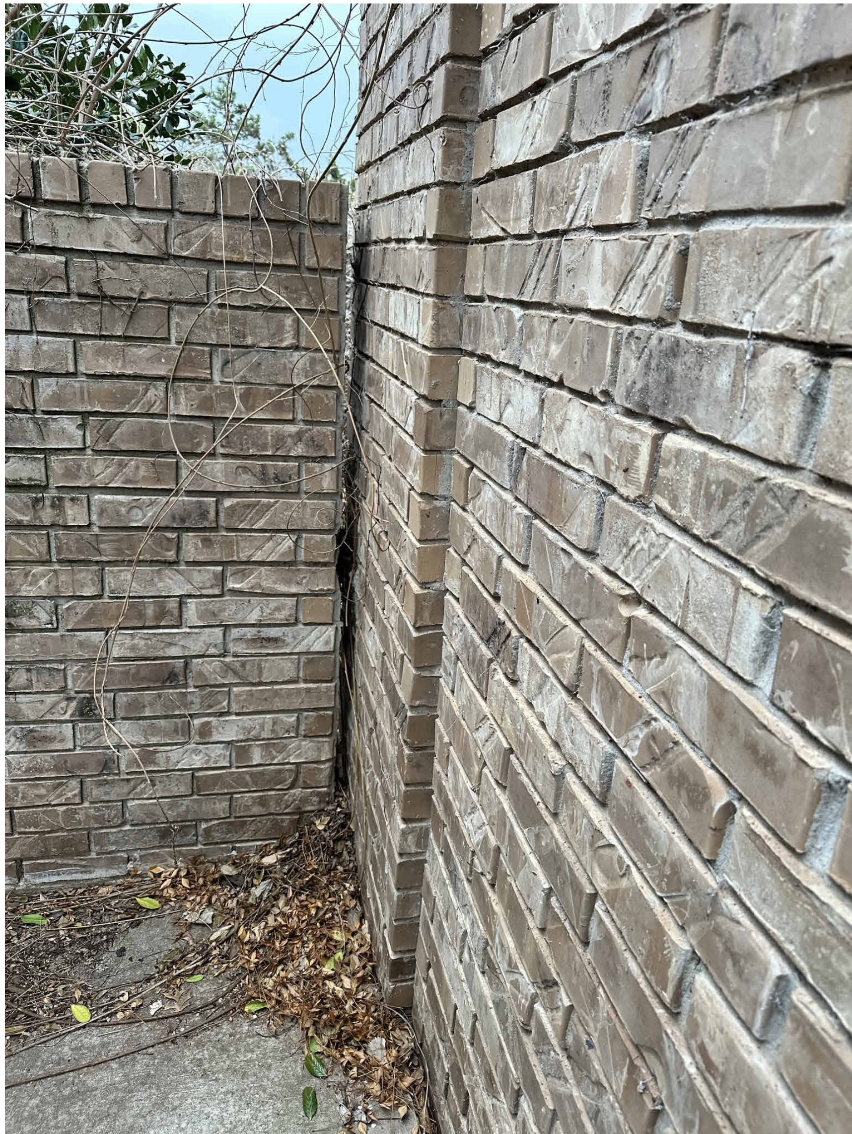
BELOW: EVIDENCE OF RETAINING WALL FAILURE AT BUILDING CONNECTION
